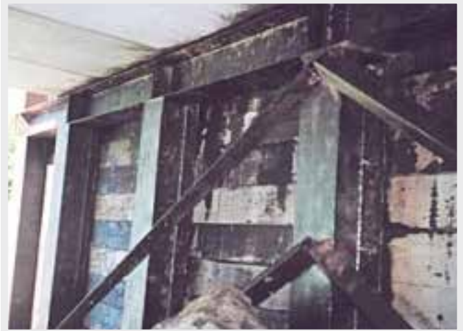
Above, the rusting has stopped. The green hue is a reflection.
